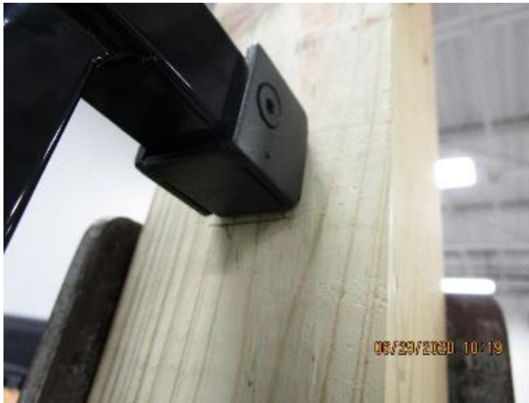
Photo No. 8 Top Rail Bracket and Connections
