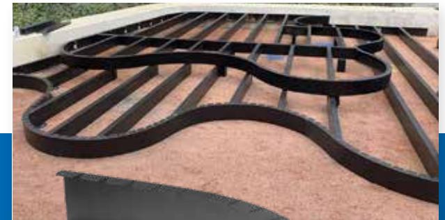
Curved Rim Joist
